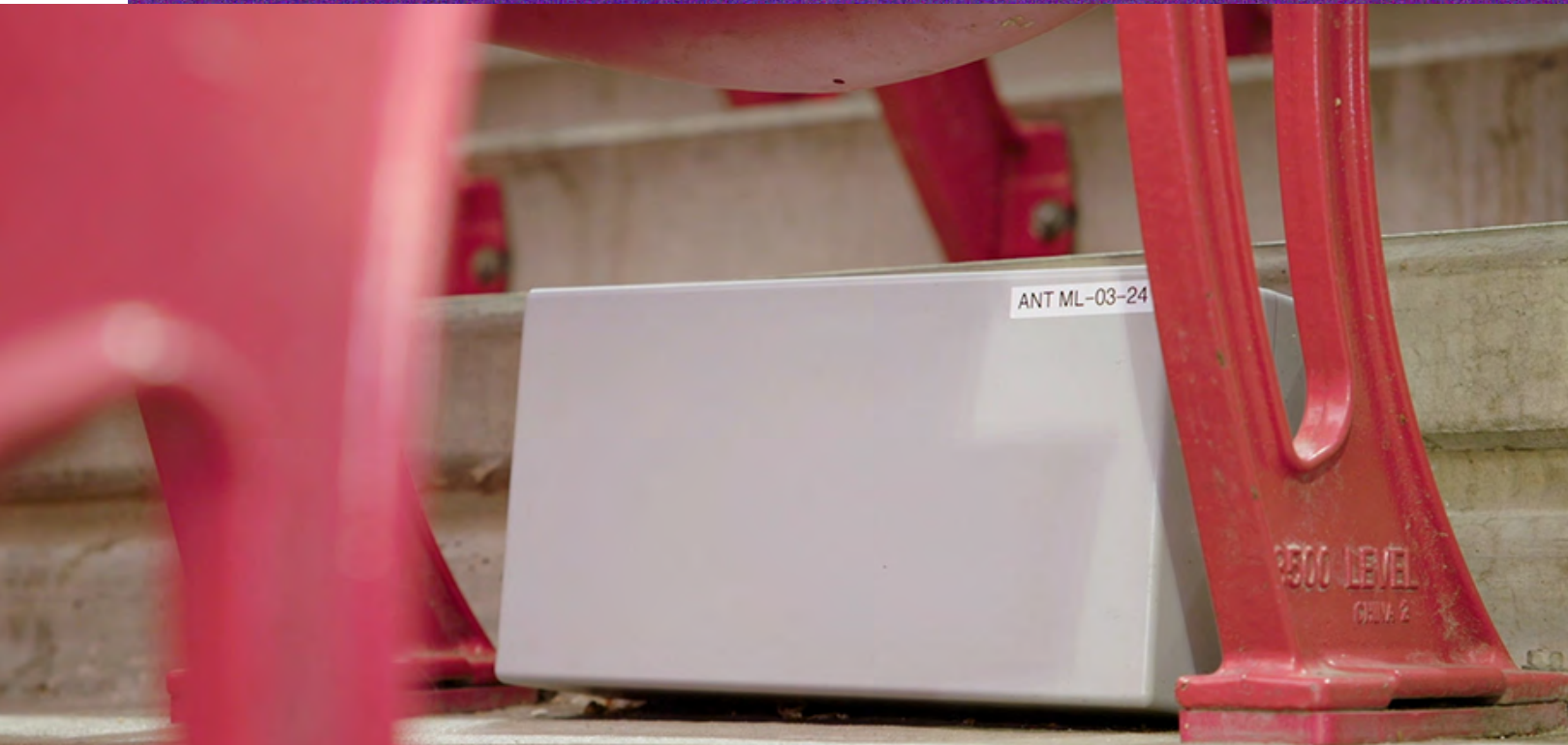
A mix of underseat (above) and overhead (below) antenna deployments were used to densify signals in all areas. Credit both photos: Verizon
