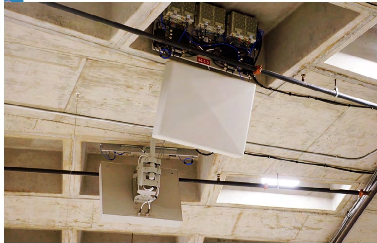
An AT&T cell on wheels (left) uses a MatSing antenna for supplementary outdoor coverage. The indoor DAS (right) supports 4G and 5G signals. Credit, left: AT&T; right: Verizon
